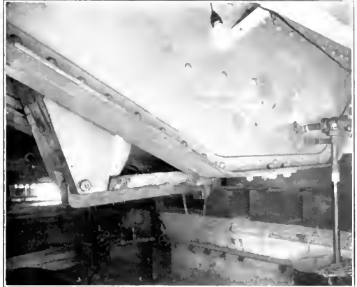
Trigger pit of the semisubmerged ways at Newport News. The trigger bears against a cast steel shoe which is located at one end of a section of the sliding ways.
